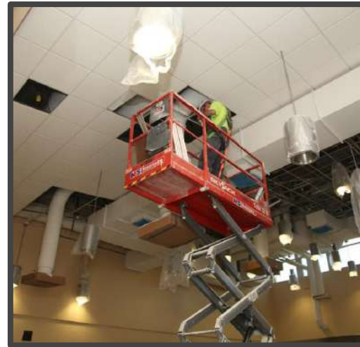
Quality installation and integration
