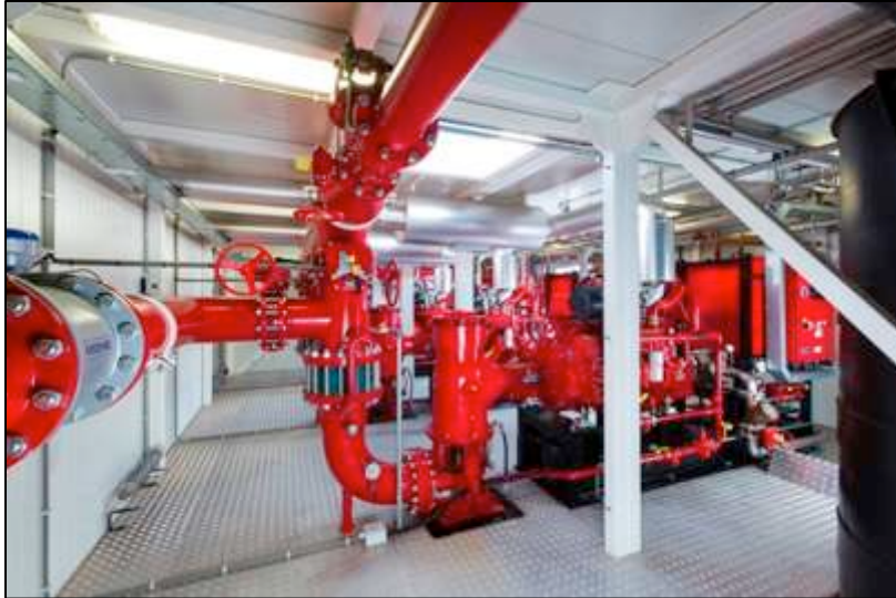
Electrical/Mechanical Rooms ASHRAE 0.42 w/sf. +
