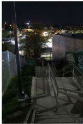
Existing pole lights off in hazardous stairwell
